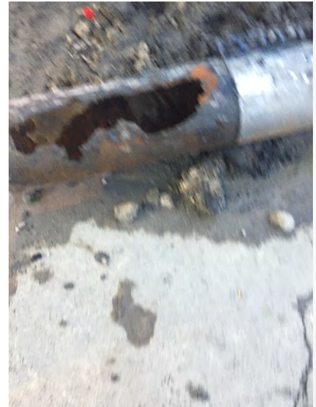
Deteriorated Pipe 3600 Block of Pratt Ave.
