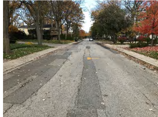
Poor Pavement – Reconstructed in 2000 N. Longmeadow Ave
