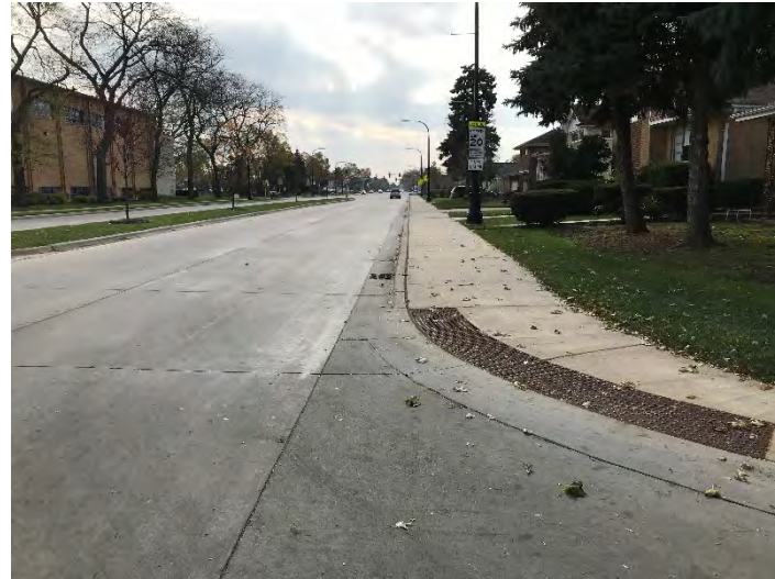
Compliant Sidewalk without Parkway N. Crawford Ave.
