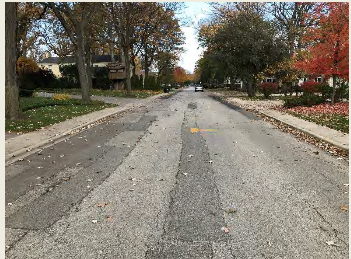
Poor Pavement – Reconstructed in 2000 N. Longmeadow Ave.
